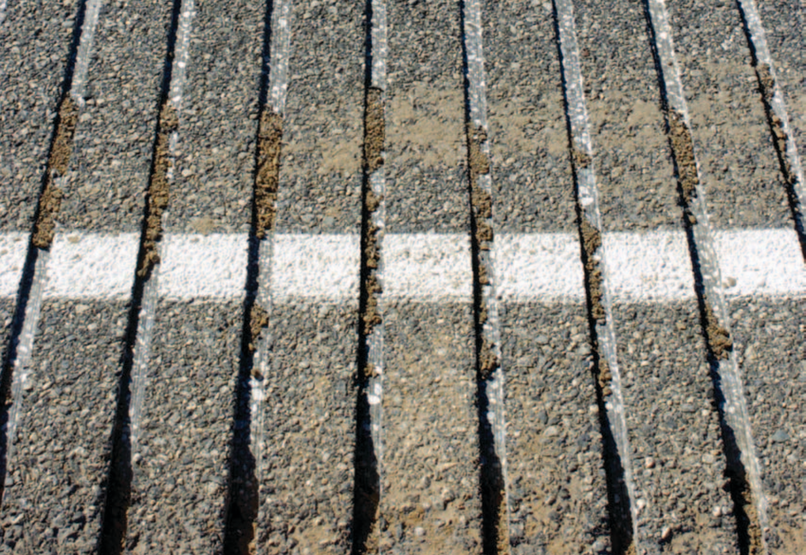
Operators created 0.5-inch-deep grooves of varying widths over a 0.25-mile stretch of road.
