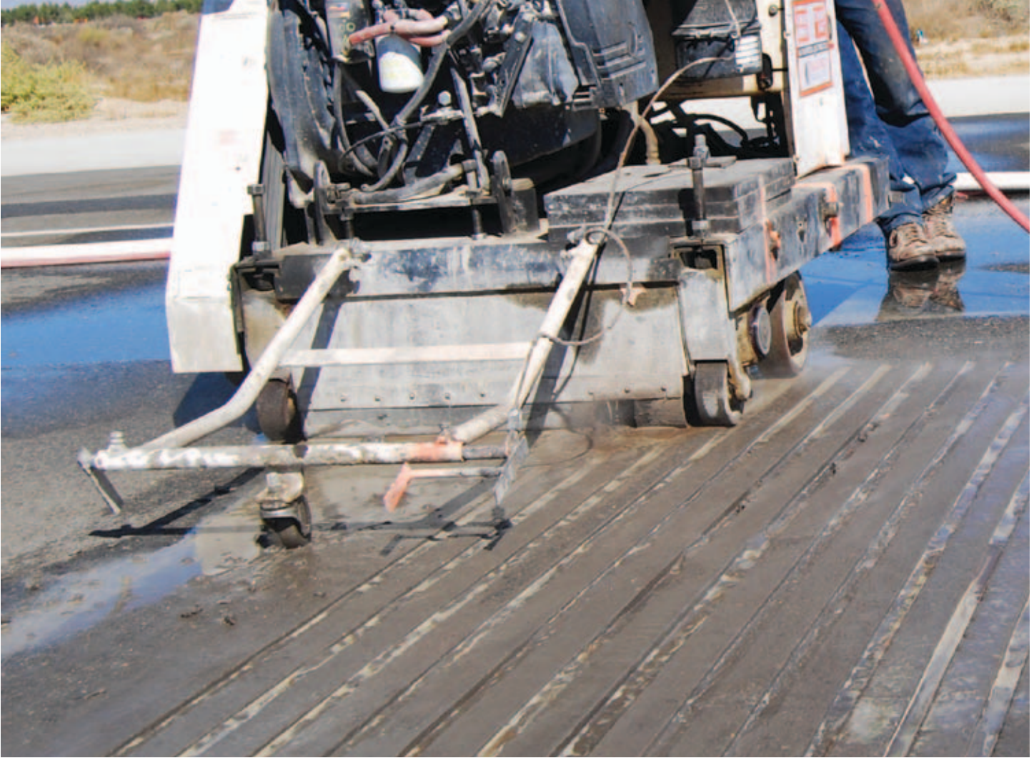
The width, depth and spacing of the grooves had to be exact.
